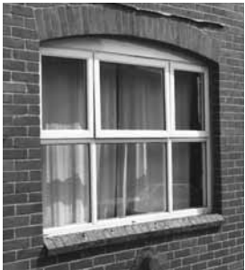
Incorrect construction using conventional DPC. Introduced in the first available horizontal run, this arrangement is suspect because it leaves a considerable amount of brickwork between window and DPC which is unprotected.
