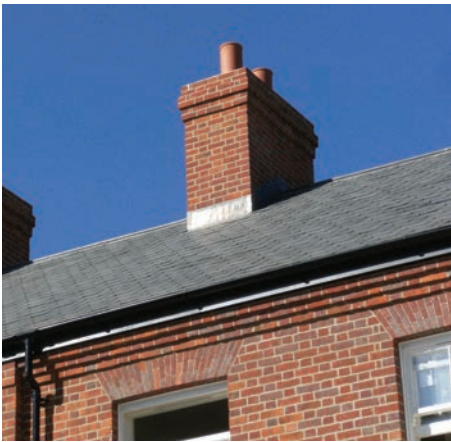
Chimney stack showing lead work. Also shown at lower level is brickwork corbel where airflow to the roof space is provided via a discreet corbel ventilator – see Ventilation section for details
